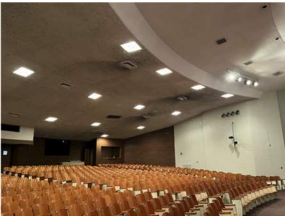
Fig. 16: Existing auditorium lighting
