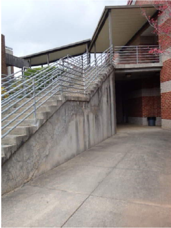
Fig. 1: Deteriorating stair, concealed entry.
