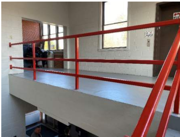
Fig. 13: Overwide gaps at too-short stair rails
