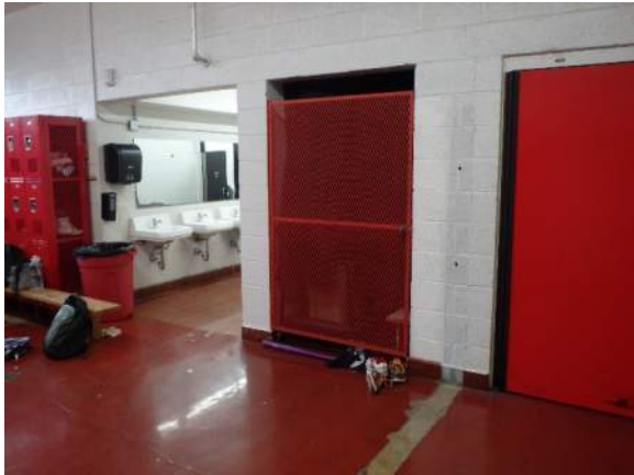
Fig. 10: Deteriorated flooring at locker room.
