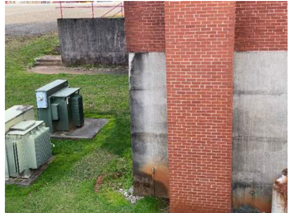
Fig. 7: Wall damage, lower level of Gymnasium.
