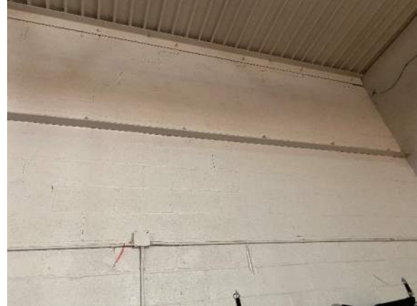
Fig. 3: Cracking at load-bearing CMU
