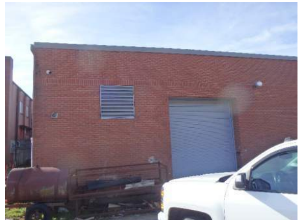
Fig. 4: Cracking at door & window heads.
