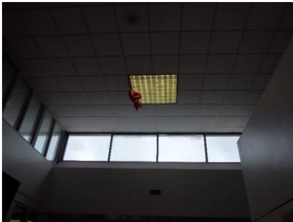
Fig. 2: Broken seals at leaky clerestory windows.
