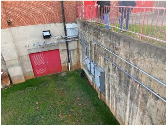
Fig. 5: Deteriorated retaining wall beside Gymnasium
