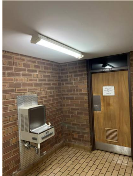
Fig. 11: Existing corridor light
