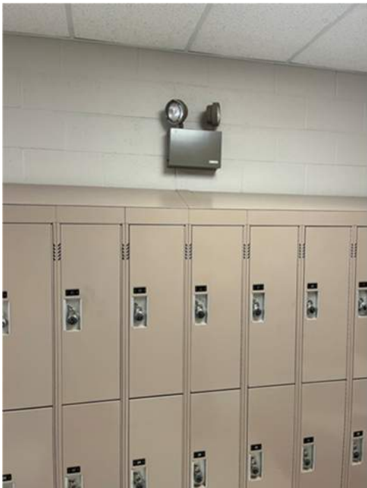
Fig. 10: Existing emergency light
