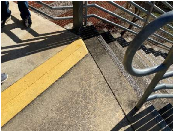
Fig. 2: Subsidence at walkway beside entry
