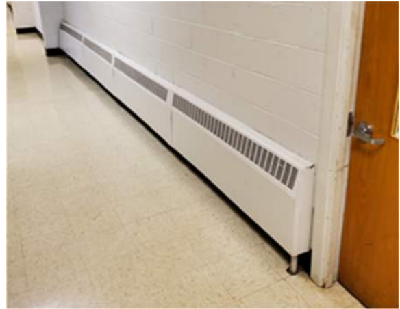
Fig. 6: Radiant heaters in hallways
