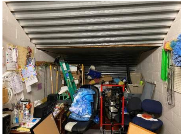
Fig. 11: Storage beneath unprotected breezeway stair.
