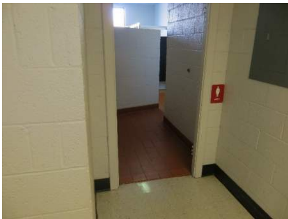
Fig. 14: Inadequate clearance, restroom entry
