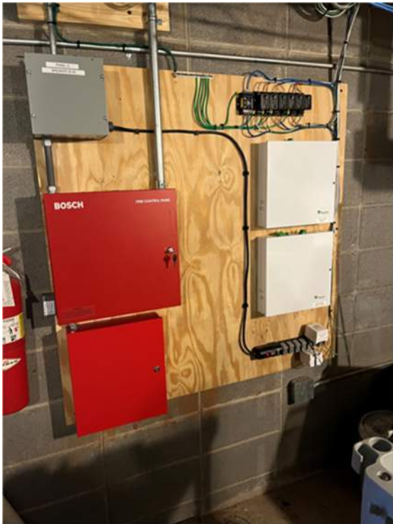
Fig. 15: Existing communications & fire alarm
