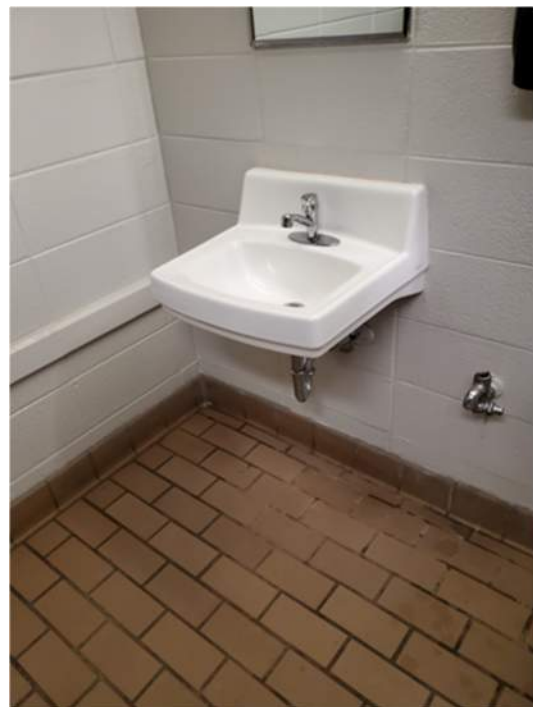
Fig. 4: Restroom fixture, stained mortar
