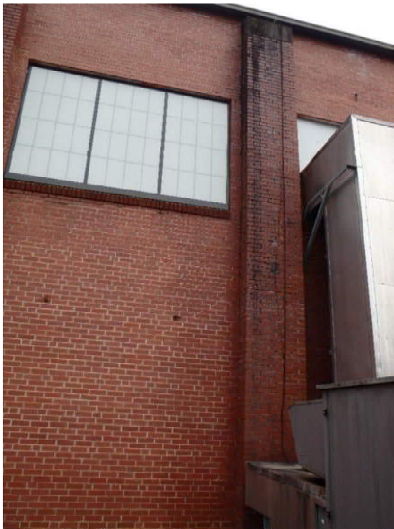
Fig 6: Extensive moisture penetration at mortar joints in walls, pilasters, sills.
