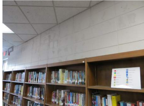
Fig. 4: Moisture infiltration at exterior walls.
