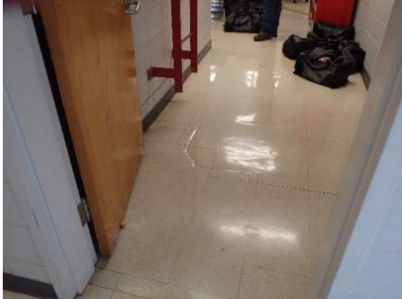
Fig. 1: Subsidence at upper level slab
