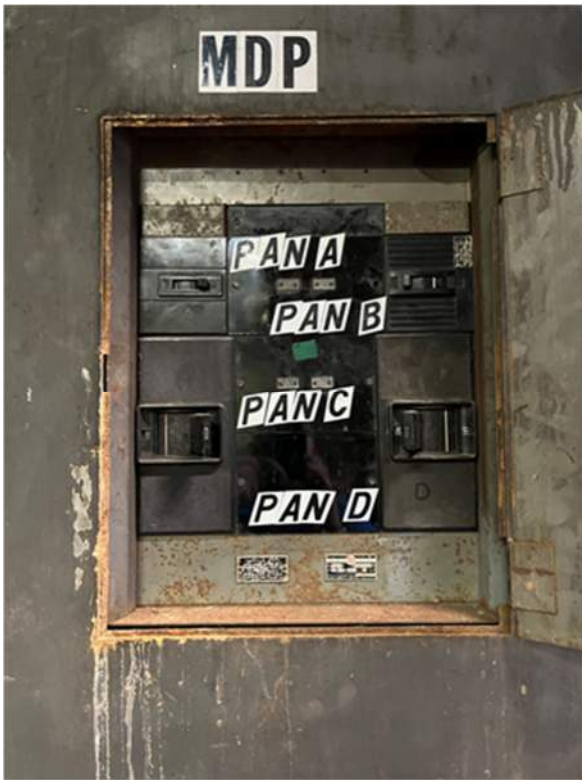
Fig. 15: Existing main panel
