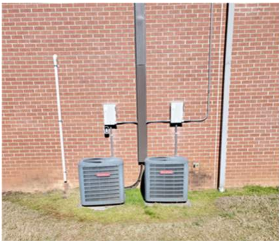
Fig. 11: Art room split system
