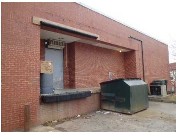
Fig. 3: Damage at loading dock; inadequate maneuvering space for trucks.
