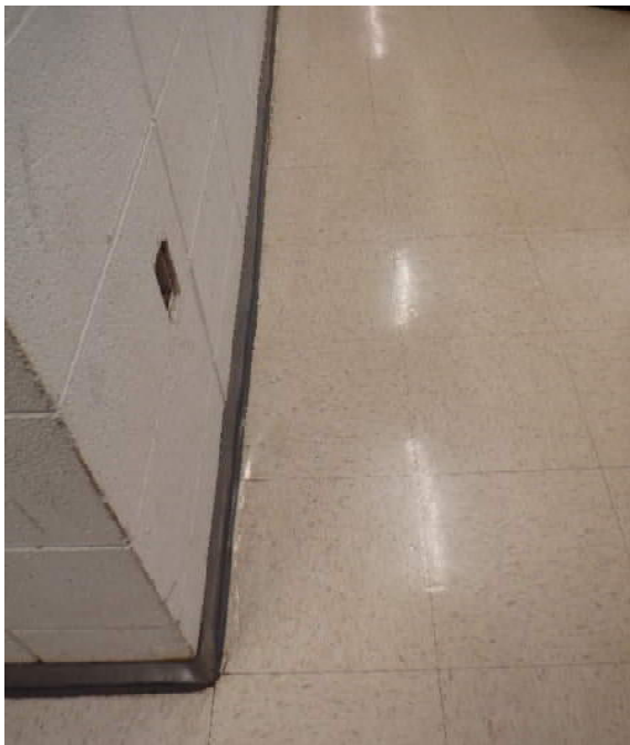
Fig. 2: Subsidence at upper level slab
