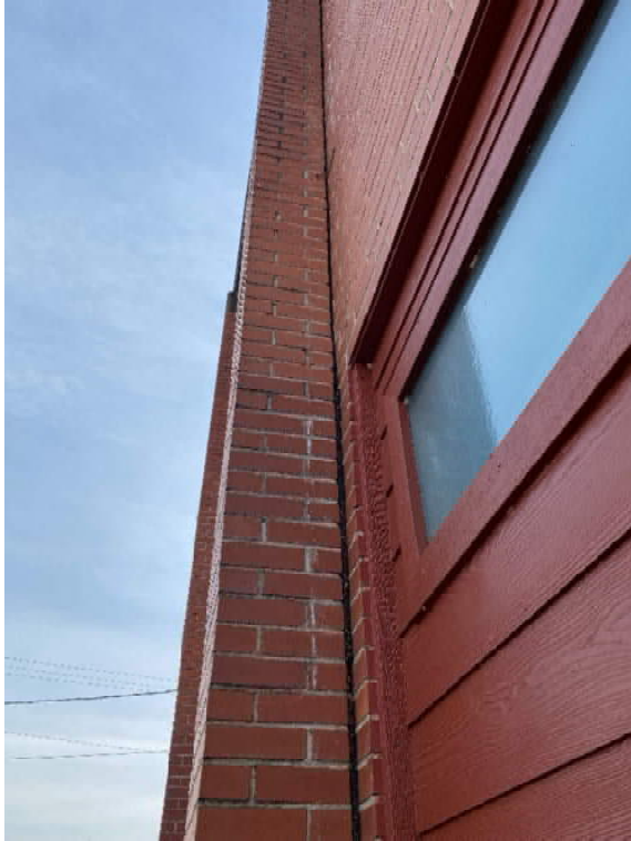
Fig. 1: Plumb bob showing extent of bowing at pilaster
