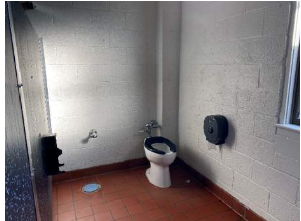
Fig. 15: Retrofit HC stall, no grab bars.
