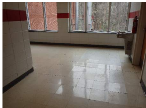
Fig. 5: Damaged VCT, upper level.
