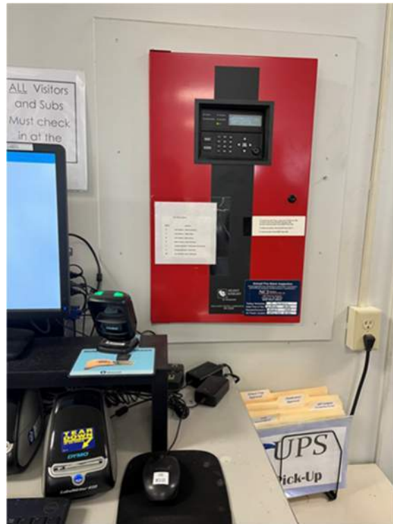
Fig. 11: Existing fire alarm
