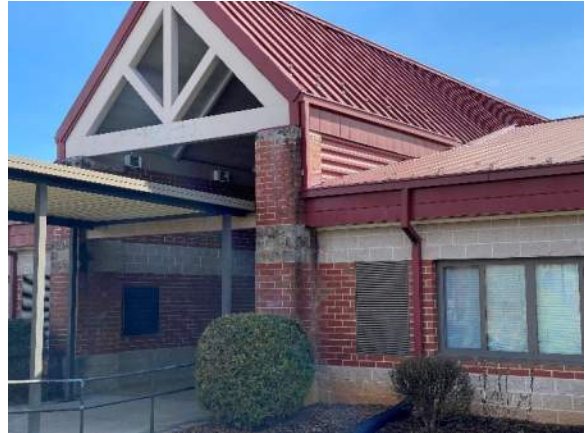
Fig. 3: Area of roof leaks, pilaster damage beside breezeway roof.
