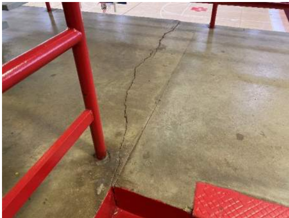
Fig. 2: Cracking at mezzanine slab
