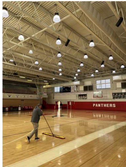
Fig. 17: Existing gym lighting
