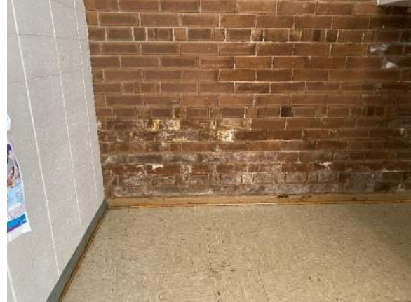
Fig 4: Moisture damage at interior walls
