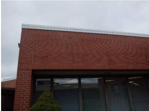
Fig. 1: Extensive moisture damage at grout joints.
