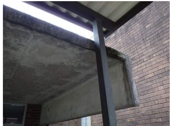
Fig. 5: Deteriorated concrete canopy
