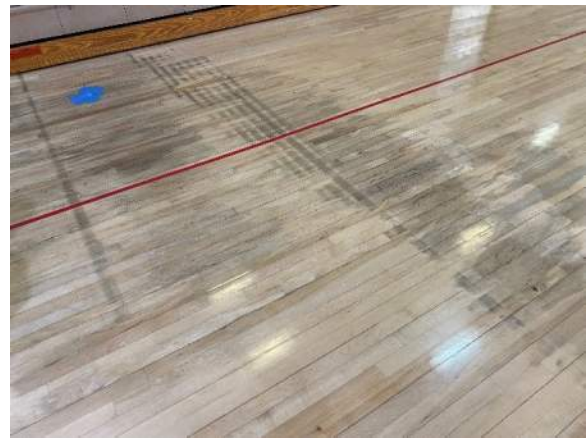
Fig. 8: Rotted gym flooring
