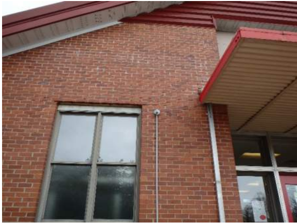
Fig. 3: Condensation in glass, rusted lintel, diagonal cracking at window head
