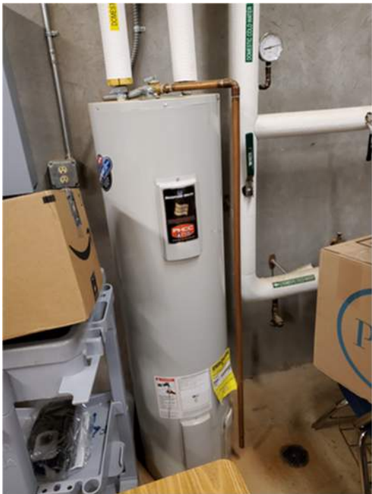
Fig. 6: Existing water heater
